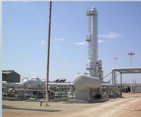
An Amine Capture Plant on a Gas Processing Plant Photo provided by CONSOL Energy
