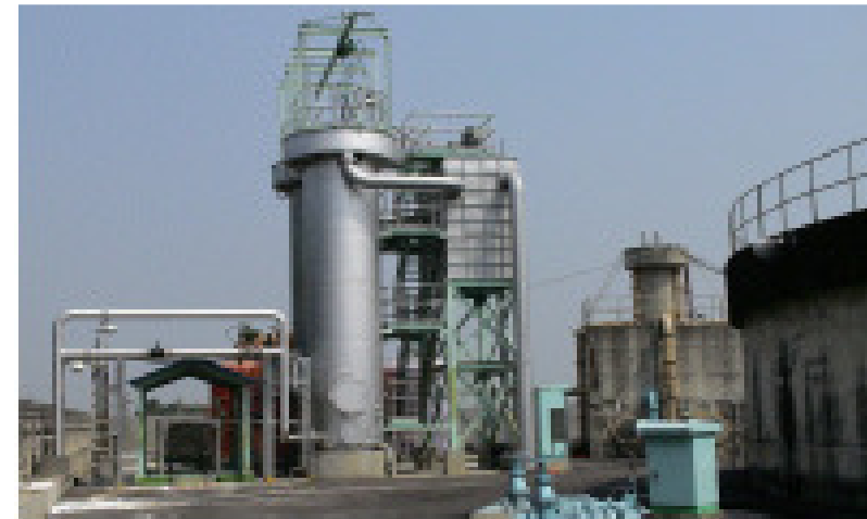
8000 m 3 /d FBC water softening project for Taiwan Water Corporation
