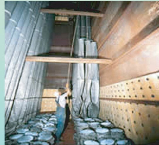
Inside of Baghouse
